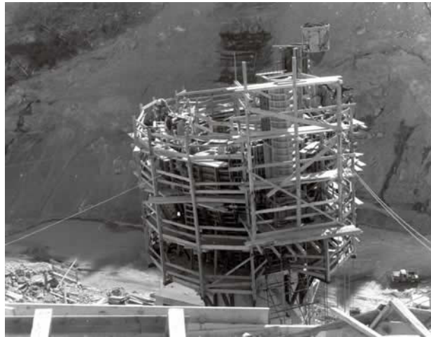
Photograph 5. Placing concrete in the spillway shaft intake structure at Joes Valley Dam (1964).
